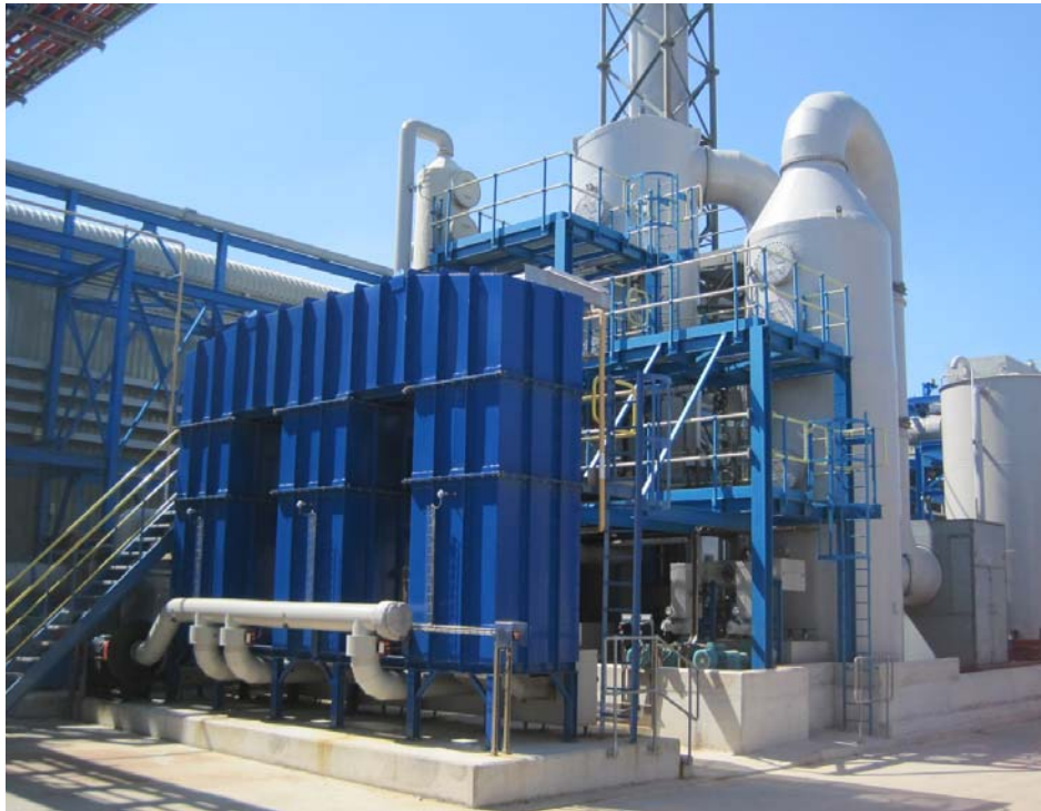
The regenerative thermal oxidiser (foreground)
