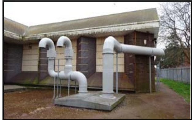
Fig 2 – Detritor extraction and air admittance dampers and ductwork and screens area
