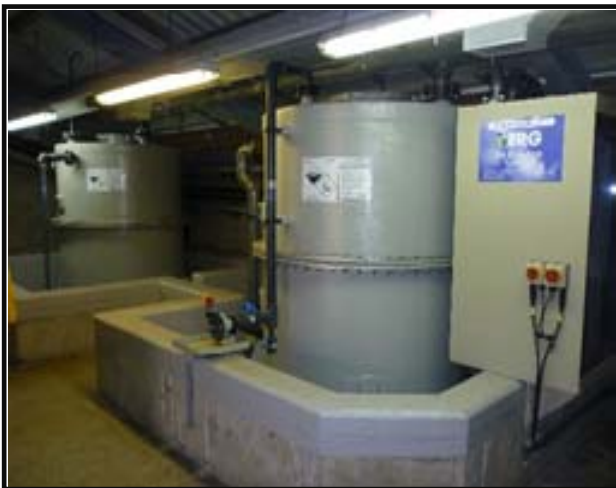
Fig 8 – New bleach tanks in the chemical store
