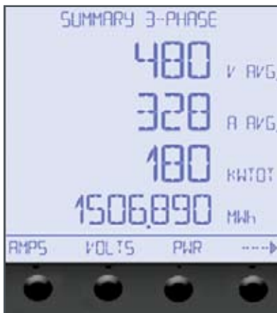
Front panel display showing function selection buttons and 3-phase voltage, current and power summary display.
